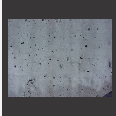
Defective Casting Repairs
